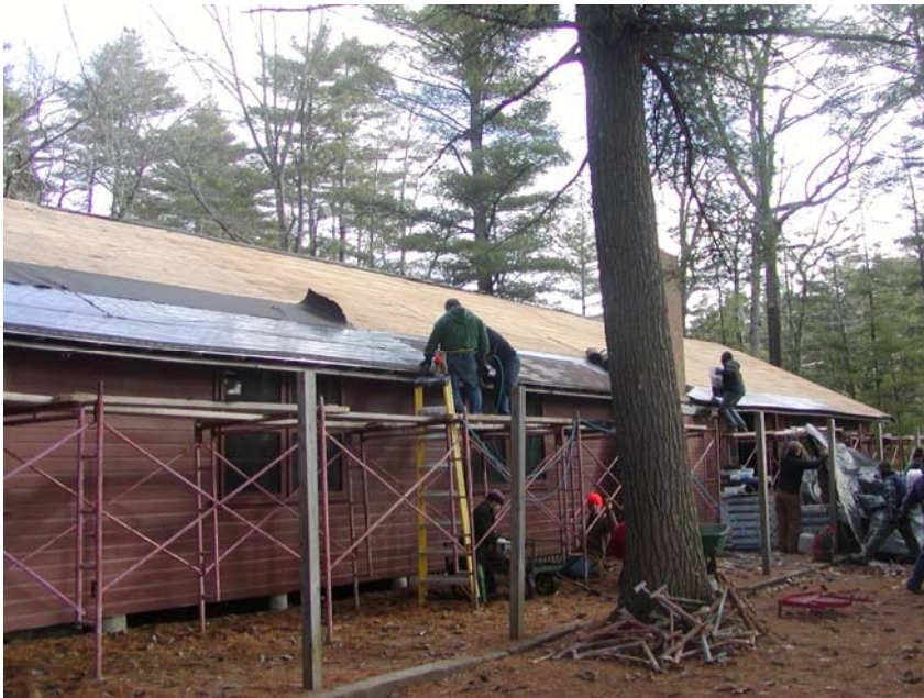
Volunteers work to put a new roof on the dining hall at Camp Hinds!
